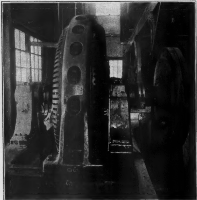
One of the Synchronous Motors
